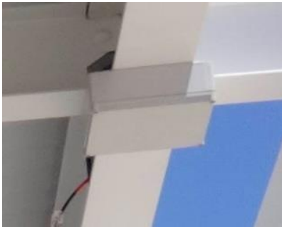
Figure 9: AP1321 with NEMA enclosure mounted on catwalk-type support
