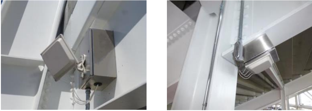
Figure 8: Directional AP1322 with NEMA enclosure on catwalk-type support
